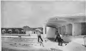
The finishing touches were being put on the strikingly-designed new market stalls when this picture was taken. The stalls will be in business this month.
